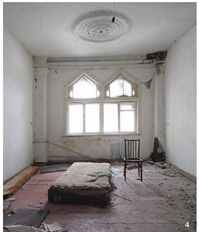
4 Tomsk: The Soldiers' Synagogue, upper floor (the former women's gallery, now subdivided into rooms) with original ceiling, windows and pillars.
